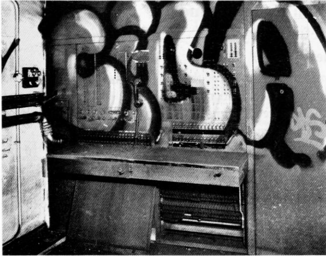
The floodgate control is now covered in graffiti. Photo Nick Catford
